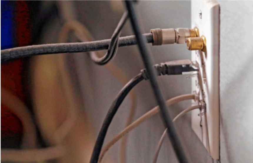
Cables connecting phone, cable and Internet service come out of a wall connector in this photograph taken last year. The Baker administration continues its review of plans and money for the "last mile" broadband effort. (AP Photo/Elaine Thompson)
